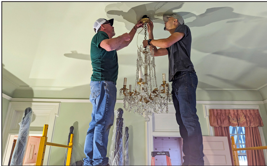
Oak Grove Restoration Co. removes the chandelier in the Primary Bedroom for rewiring.
